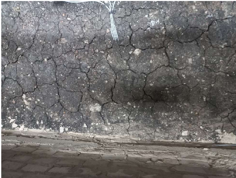
Figure 4.10: The north-facing side of the expansive clay soil
