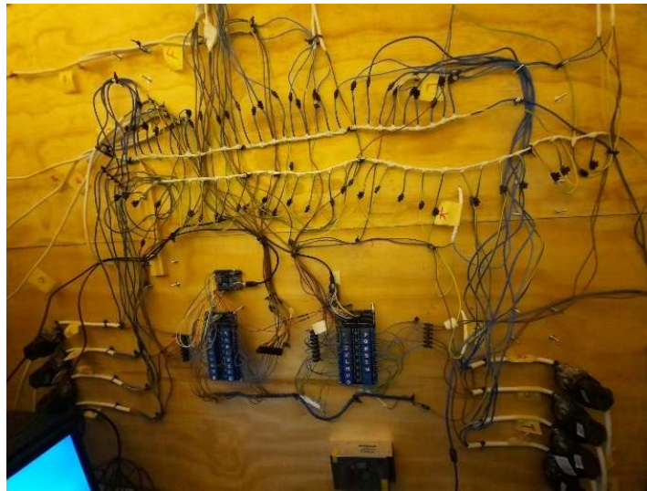
Figure 3.10: Photograph of the circuit of heater lights
